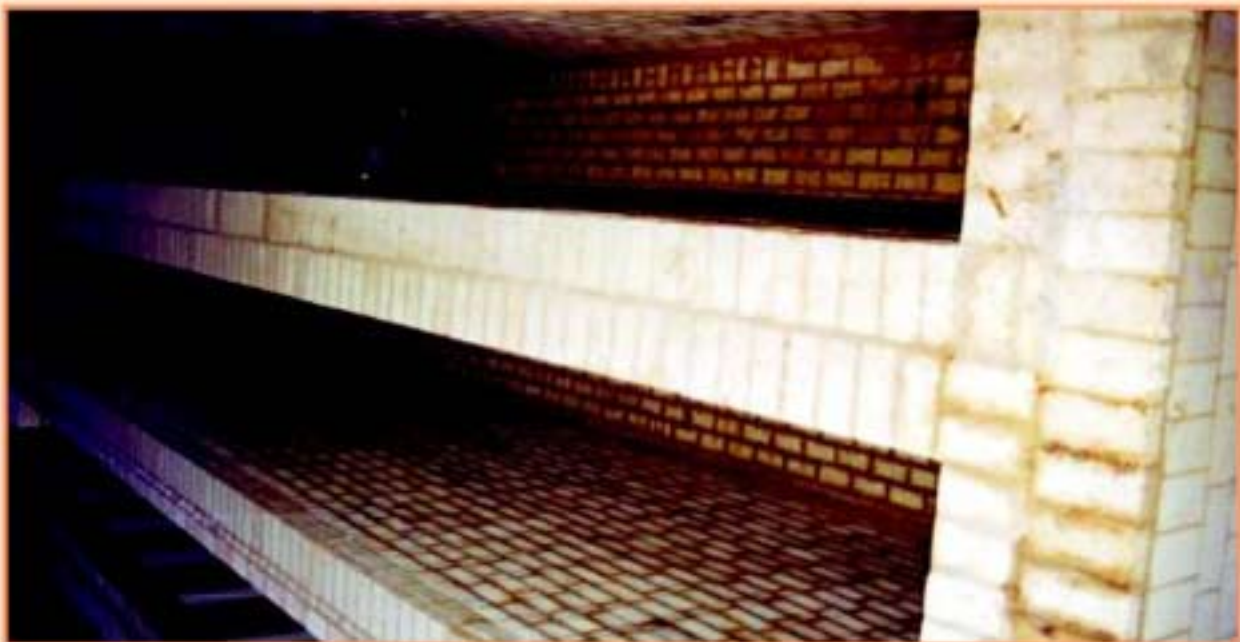
ACID PROOF BRICKS LINING FOR GALVANIZING TANK
