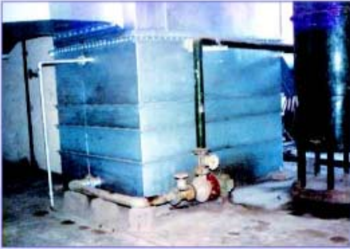
MS / FRP LINED EQUIPMENT
