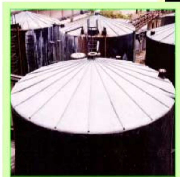
CYLINDRICAL VERTICAL STIFENED CONICAL TOP TANKS
