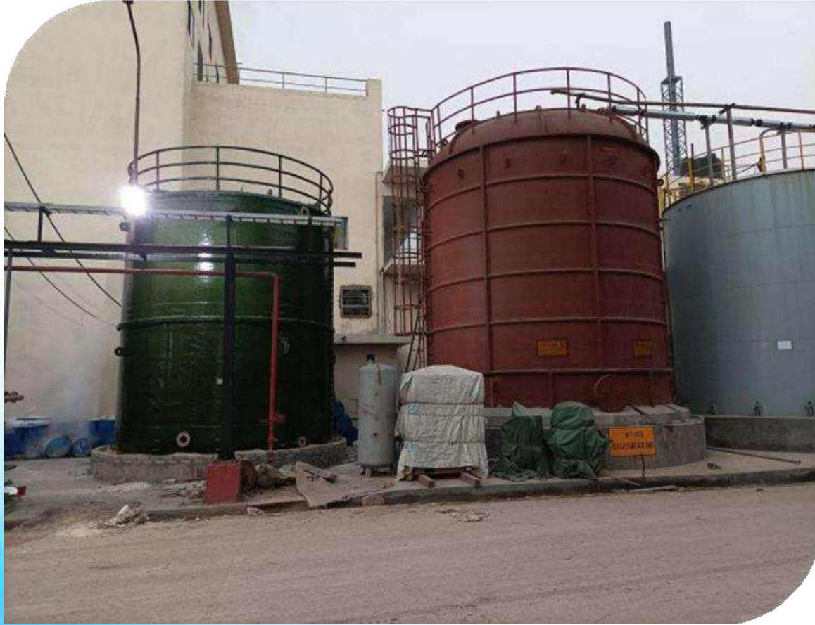
SULPHURIC ACID STORAGE TANK - BANGLADESH
